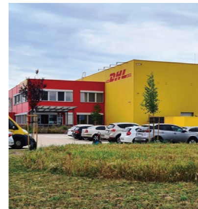
Airport Bratislava, Slovakia. Logistic Depo DHL Big capacity duct units for heating
